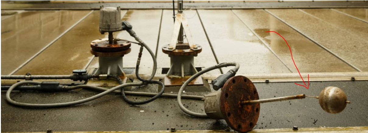
{A bent arm of the float switch.}
